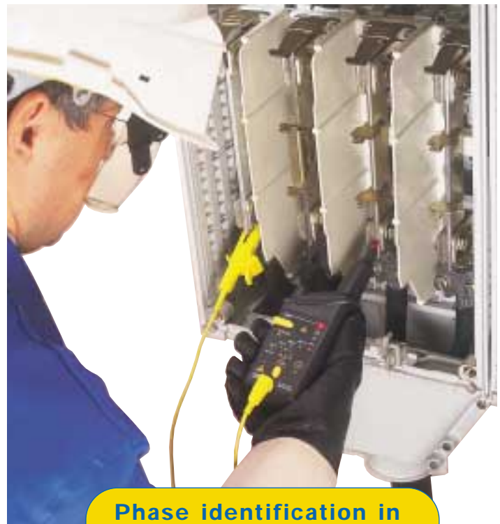
Fuse continuity test.
