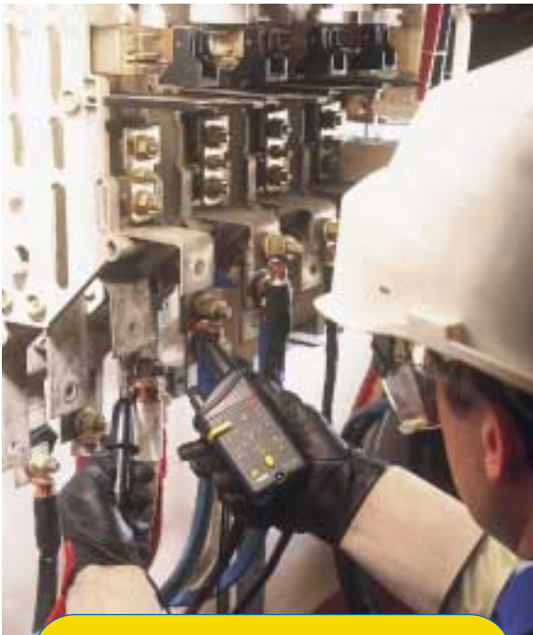
Phase rotation test in a low-voltage panel.
